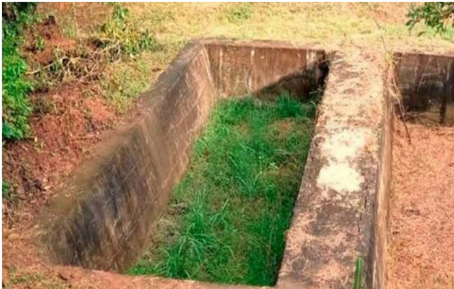
Fig. 10. Barichara WWTP drying beds. [13]
