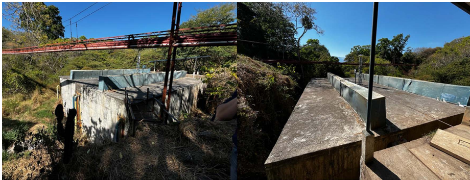
Fig. 5. Status of Wastewater Treatment Plant (WWTP) of the municipality of Barichara. [8]
